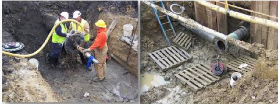
Insertion of ILI tool into Pipe Segment
